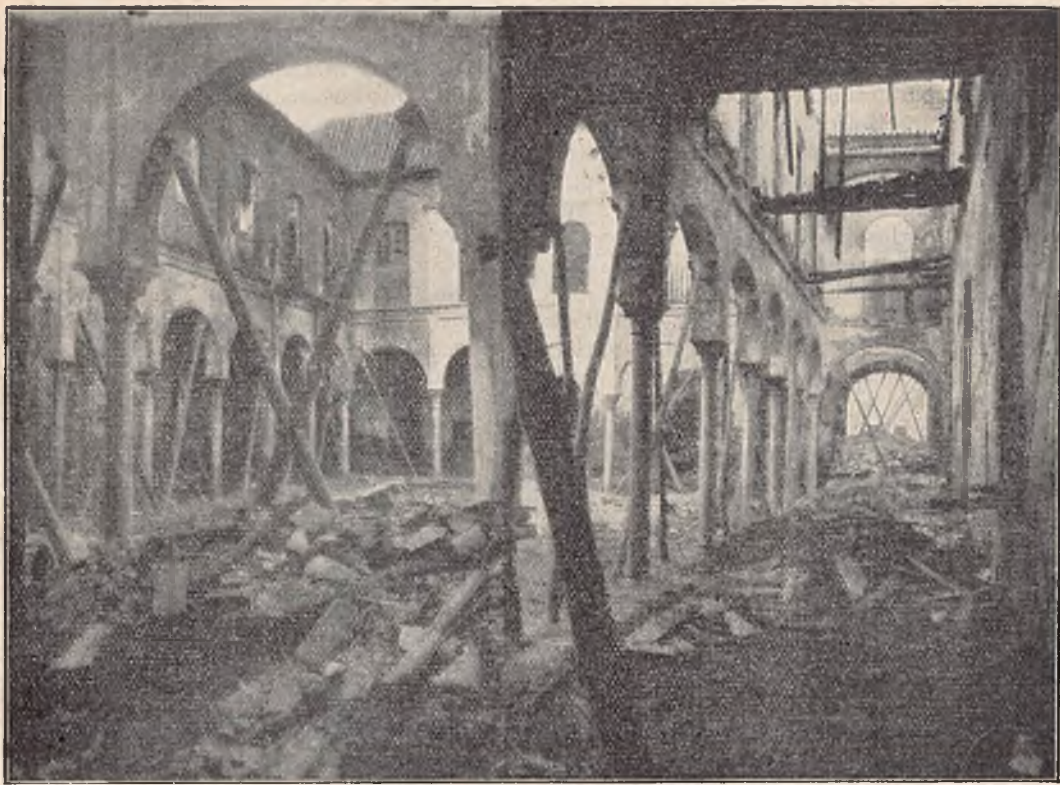
Seville. Spain. — The scene after the fire that devastated the Salesian School - p. 2.
