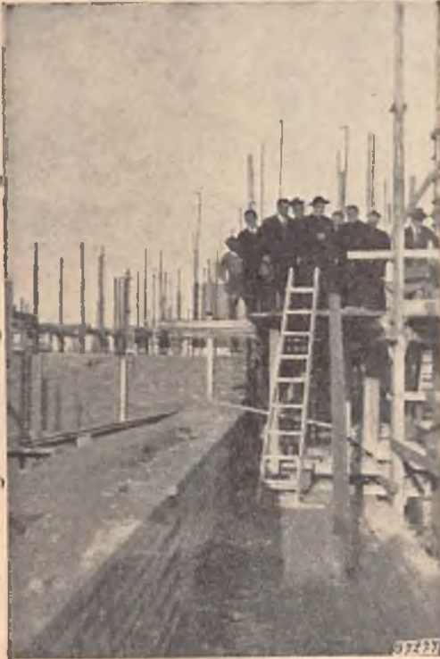
Rome. — The Superior General inspecting the work on the new Church of Our Lady, Help of Christians.
