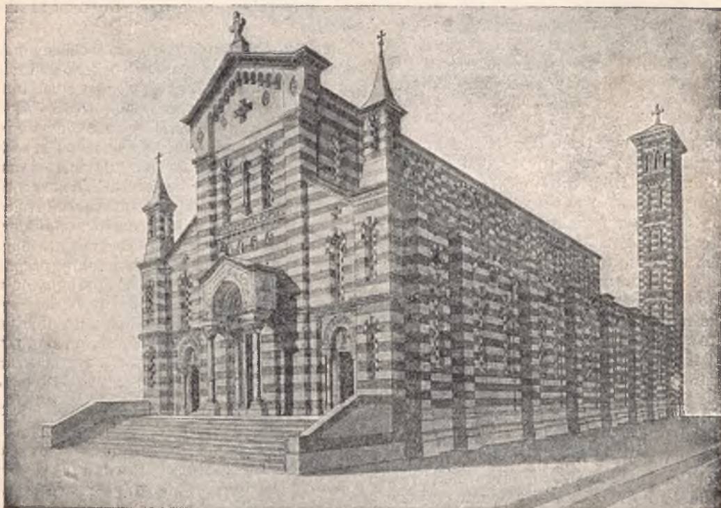
Salesian Church of our Lady of Snow in course of erection at Spezia.
